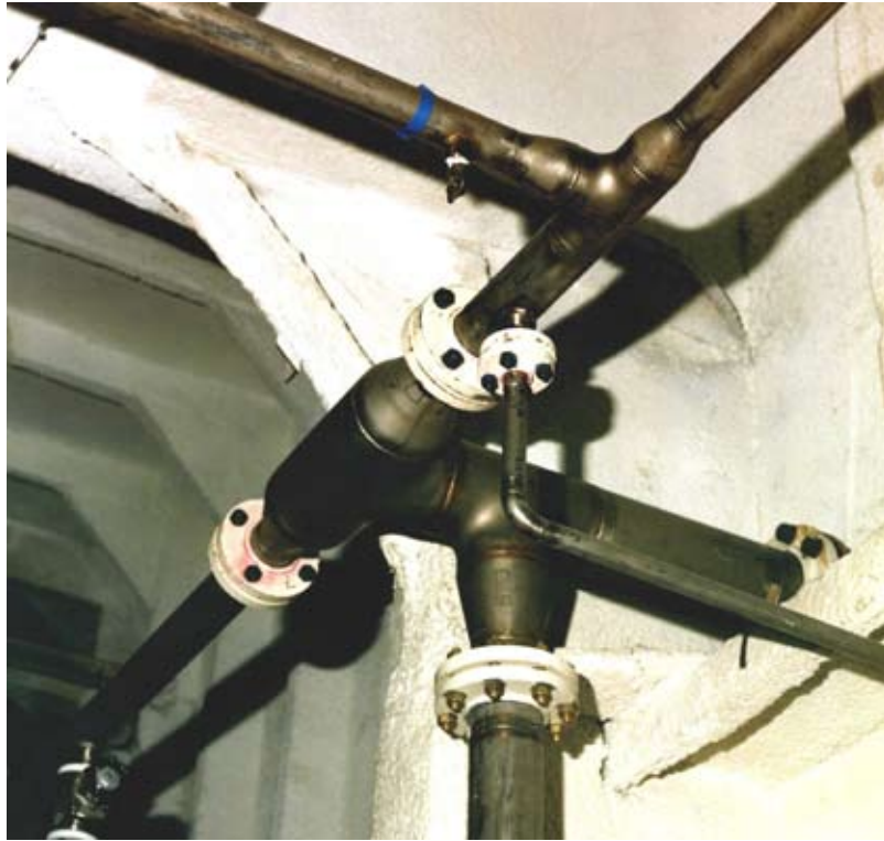
FIGURE 11 Replacement Zeron 100 firewater system on Mobil Beryl 'A'.
