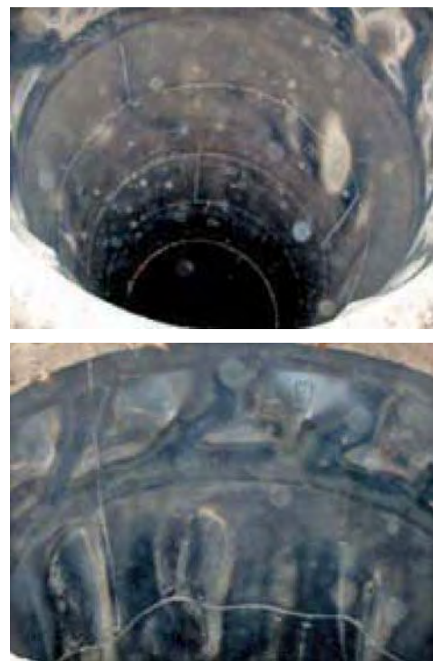
Fig. 3. On top, an RA 253 MA dip tube after six years in service at 1600°F. On bottom, distortion in a dip tube that was typical for 310 stainless after two to three years of service. Dip tubes are 8.5 feet in diameter and 23 feet long and hang vertically.
